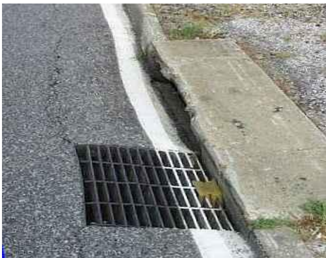
Figure 16. Catch Basin http://www.neponset.org
