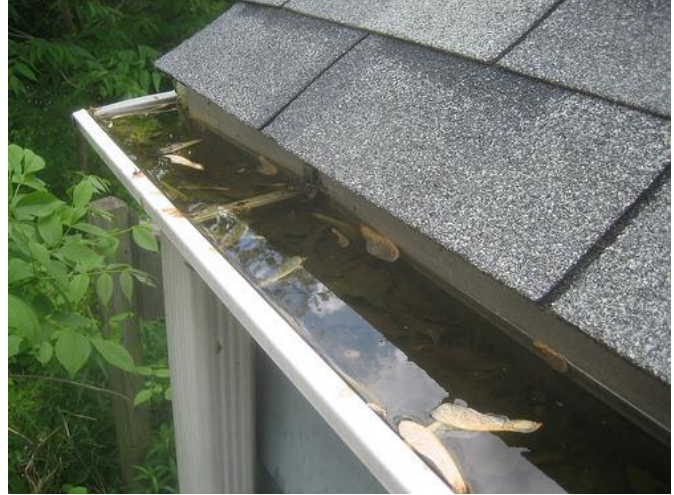
Figure 19. Clogged rain gutter filled with water ( http://www.moonworkshome.com )
