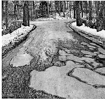
(a) Pavement condition of Goodhue Street from the town line towards Waldingfield Road.
