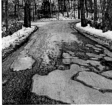
Figure 12a Existing Pavement Condition on Goodhue Street
