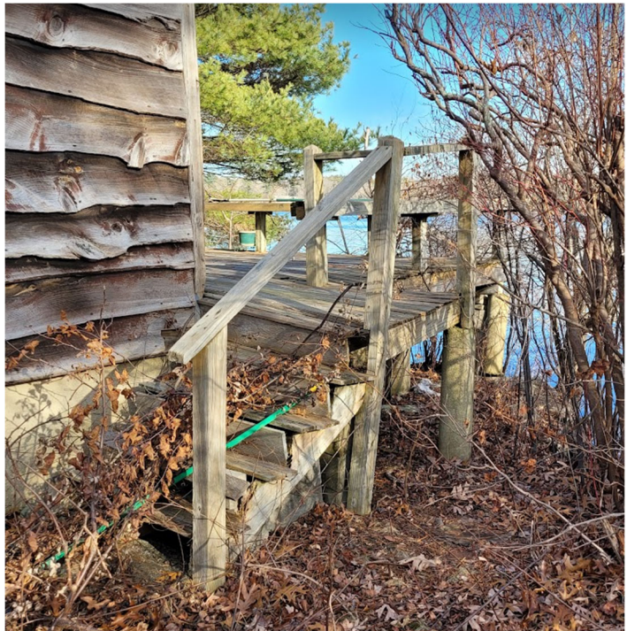
Photo of the existing deck and stairs to be removed and replaced with a new deck and stairs supported on helical piles.
