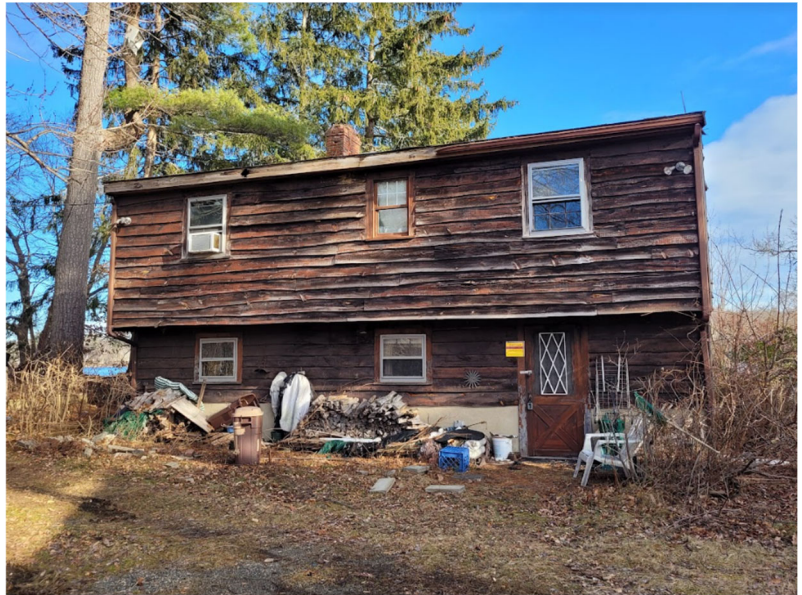
Photo of the existing single family home to be renovated within the same footprint and a second story added. The first floor is a walk out basement, and second floor is the first story in this photo.
