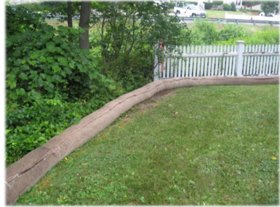
Example of Groundscapes Filtermitt used as sedimentation control at typical residential project site.
