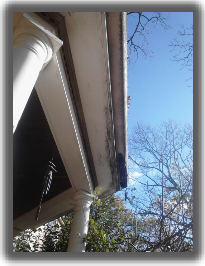
7 Year Old Wood Gutter -Arlington, MA
